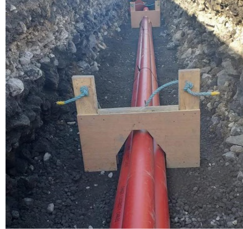
Figure 2: A typical cable duct installation in the road
