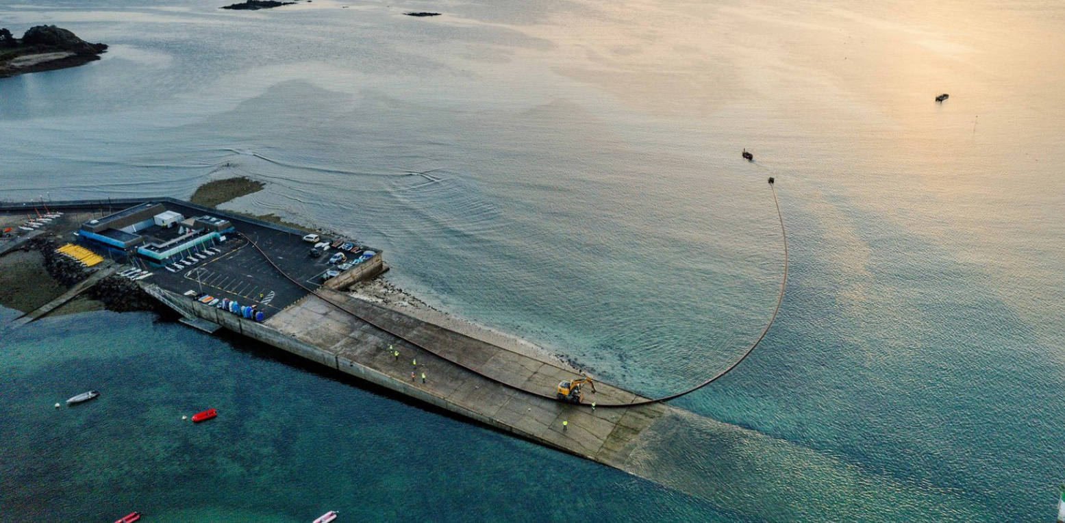
An aerial view of the French landfall operations, including the towing of HDPE pipes.
