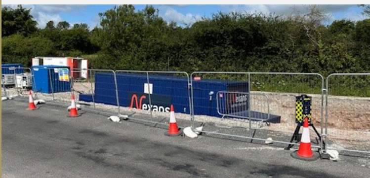
A Nexans' container in a joint bay along the cable route, inside which joining specialists join together the cable lengths.
