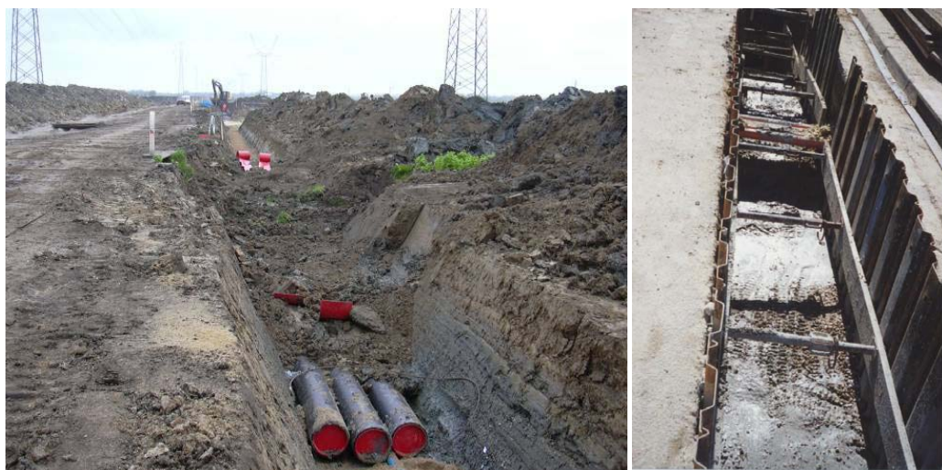
Figure 1: Cables in pipes (left) and cables in ducts (right), which are pipes cast in concrete. The pictures are examples given in Cigré TB 398.
