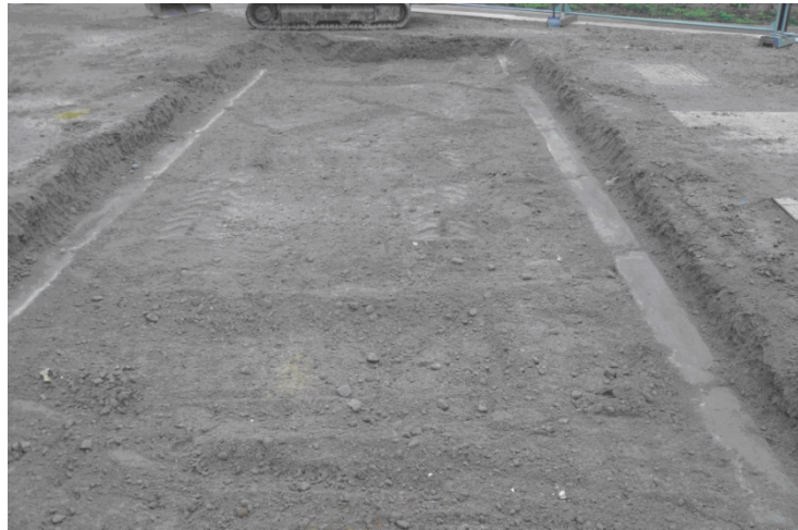
Figure 4: Soil in uncovered joint pit after a failure of 15 kA during about 50 ms.
