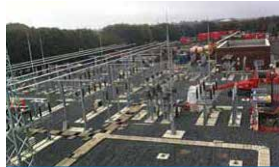
Cloghran 110kV station.
