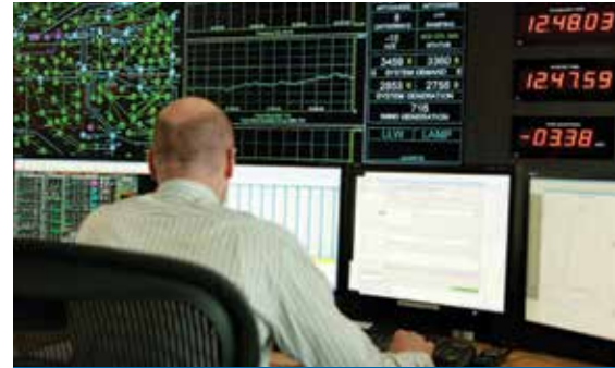
The National Control Centre, Ballsbridge, Dublin.
