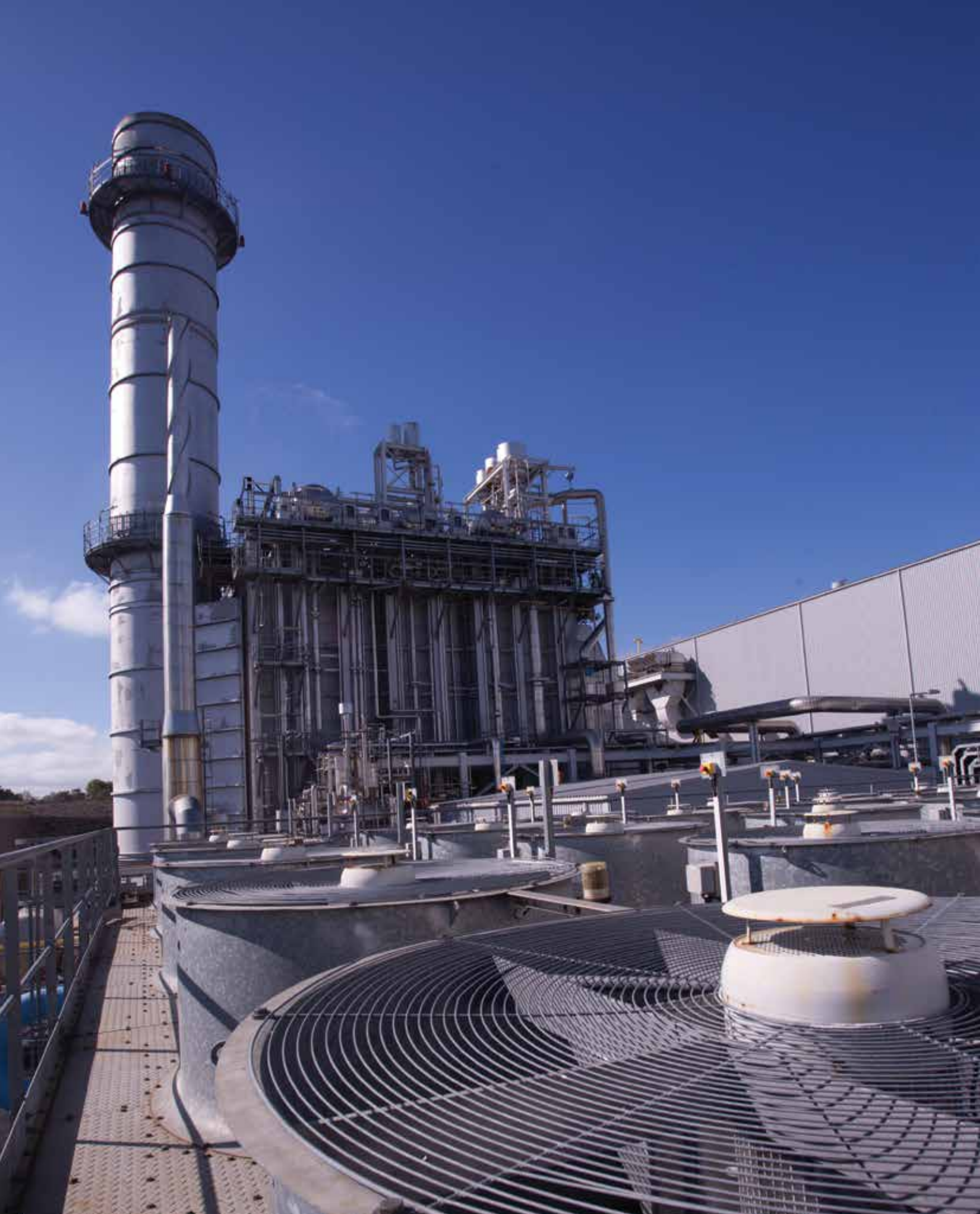
Tynagh Power Station, Co. Galway.
