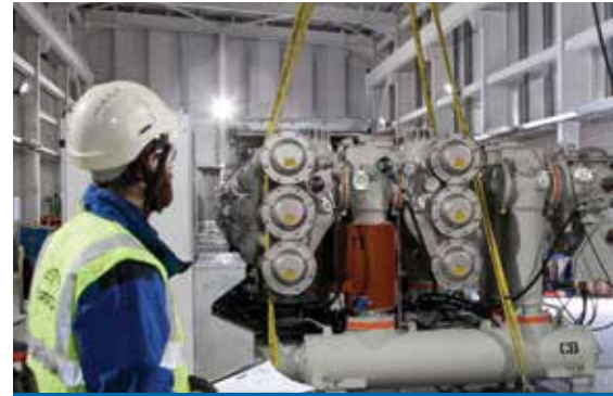
GIS infrastructure located in Tarbert station.
