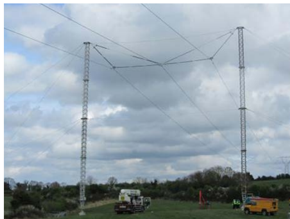
Emergency restoration system
