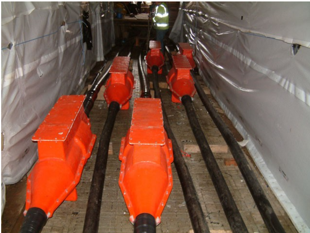
Figure 2 EHV Joint Bay Containing Six Joints
