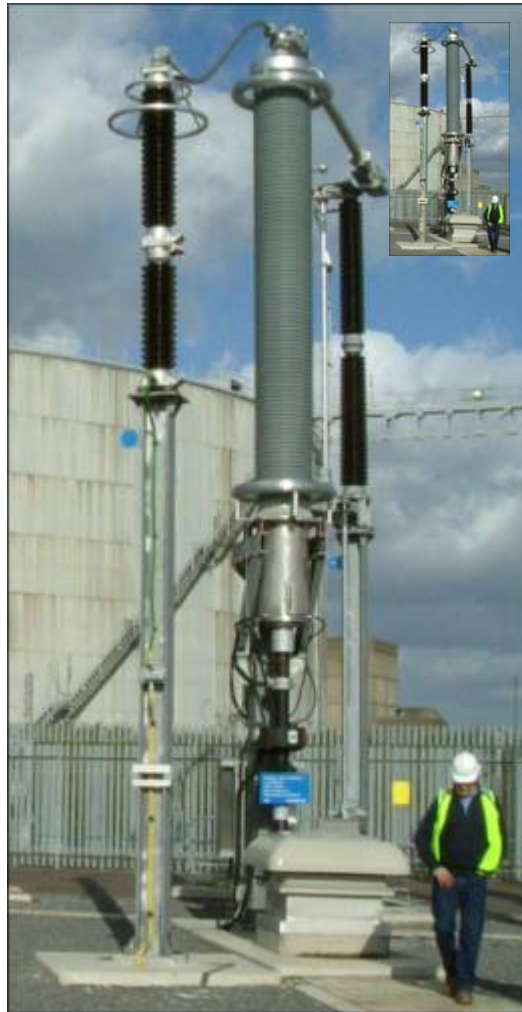
Figure 3 400kV Cable Outdoor Sealing End (ODSE) Termination
