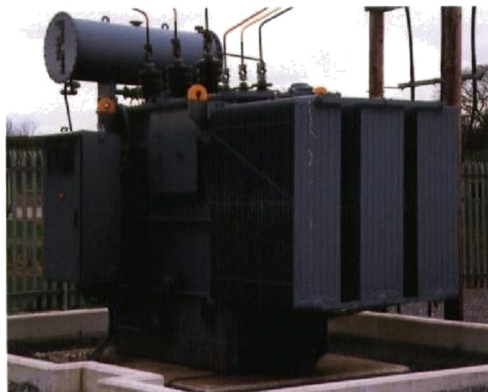
Example of a Banded Transformer
