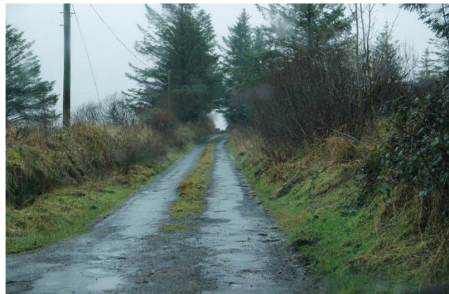
Road A: Example of narrow section in poor condition
