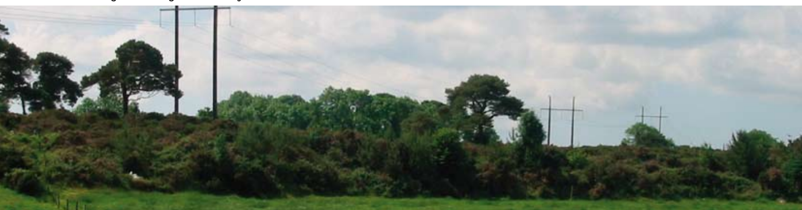
Fig.1 Existing Dunmanway-Macroom 110 kV line
