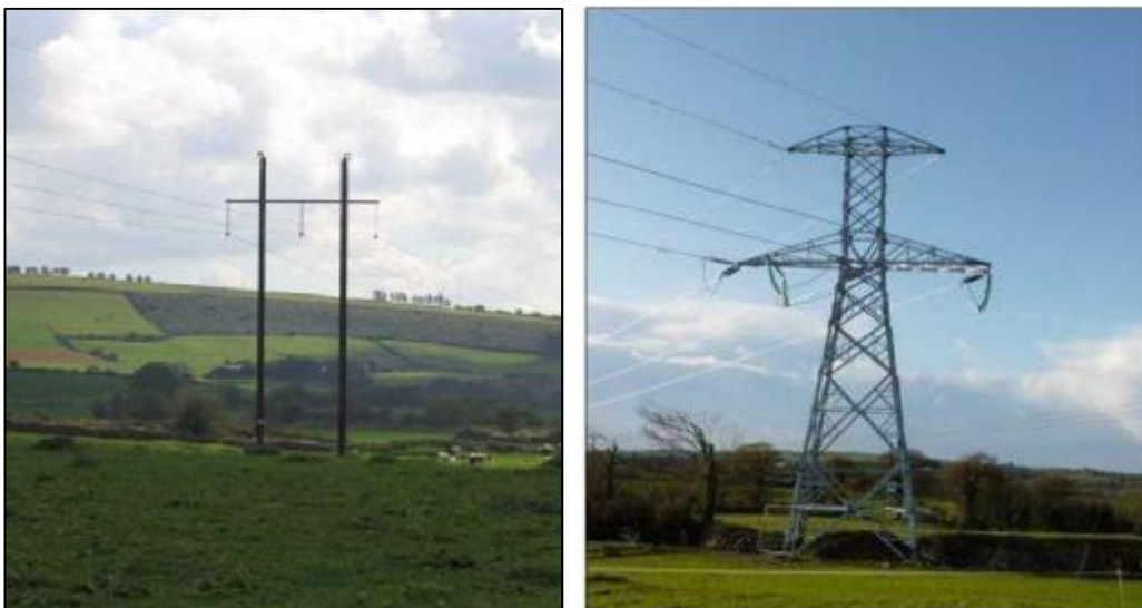
Figure 5: 110 kV single circuit poleset with shield wire (left) Typical 110 kV single circuit OHL steel angle tower with shield wire (right)
