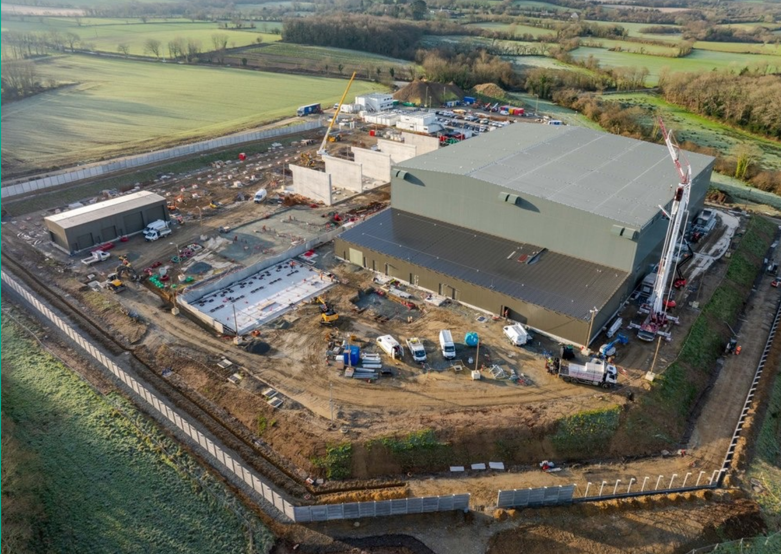
Works progressing at the Ar Merzher converter station site near La Martyre substation (Finistère) France.
