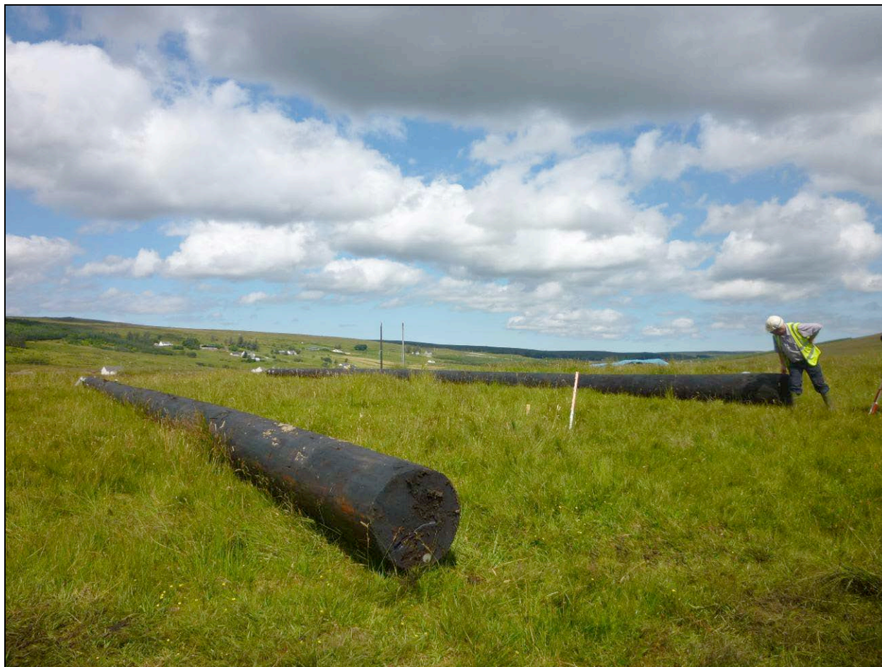
Double wooden poleset in place in advance of erection on Donegal 110 kV Project (Binbane – Letterkenny)
