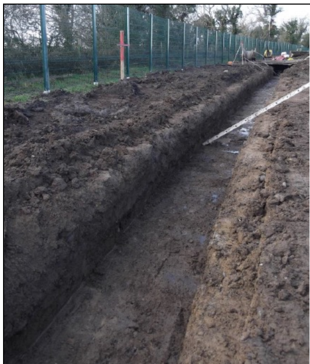
Cable trench linking substation to converter station (400 kV), East West Interconnector Project. Courtesy of Byrne Mullins & Associates
