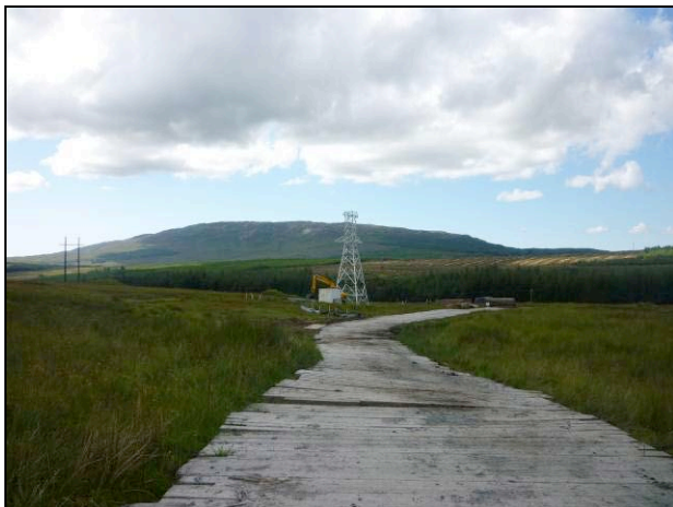
Example of a temporary access road over soft ground using aluminium panels
