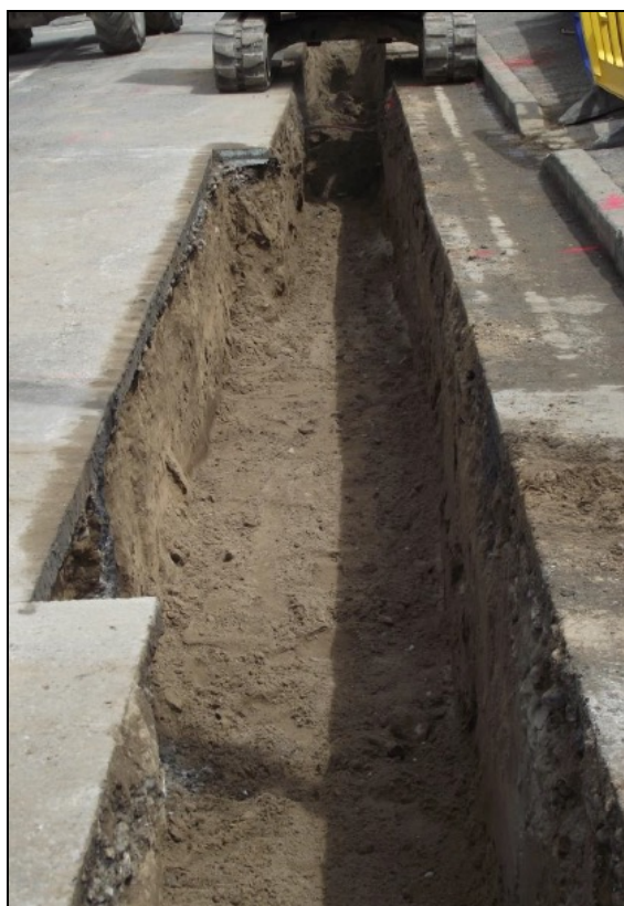
Cable Joint Bay, East West Interconnector DC UGC Project. Courtesy of Byrne Mullins & Associates
