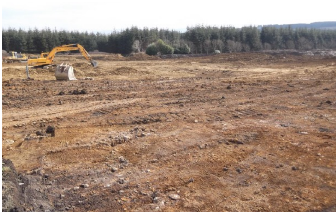
Ballynahulla (also known as the East Kerry North West Cork) Project General View Ground Preparation Works for Substation courtesy of Byrne Mullins & Associates
