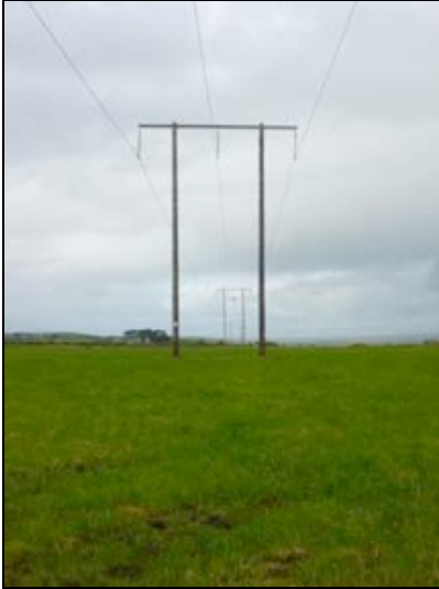
Example of 110 kV wooden polesets
