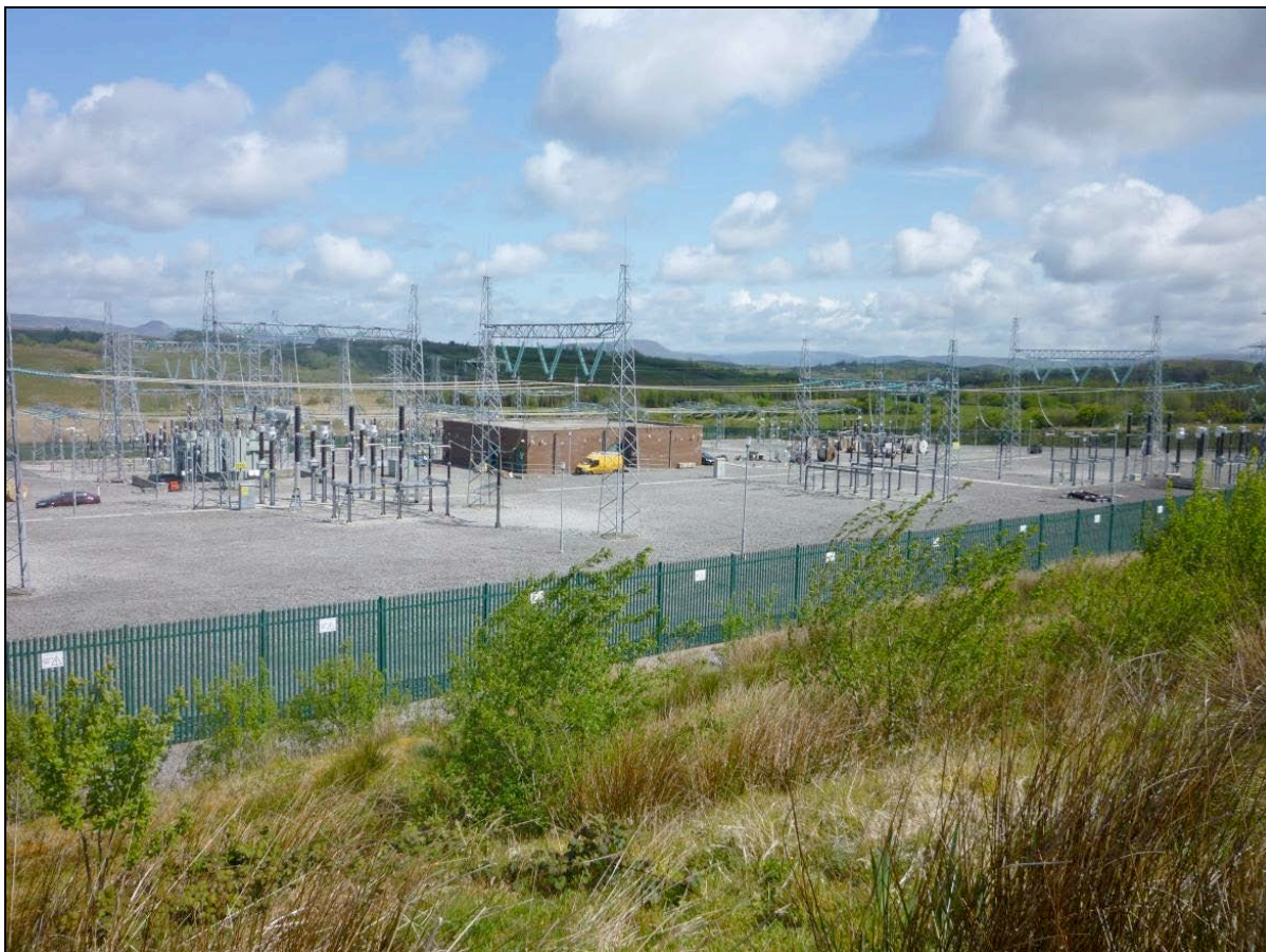
Srananagh 220kV/110kV substation, Co Sligo, example of a typical AIS substation
