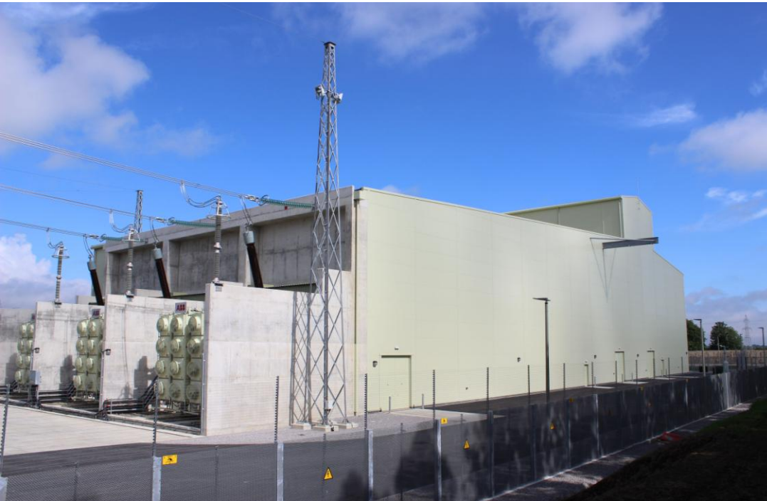
Above: The Interconnector cable terminates on either side of the Irish sea at the respective Converter Stations where the AC/DC conversion takes place.
