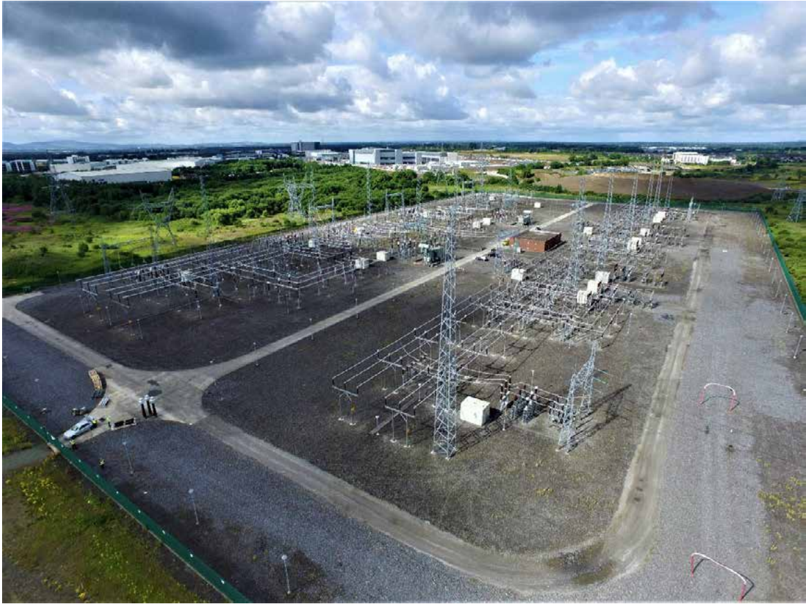
Figure 3.12: 220 kV Air-insulated substation (AIS)
