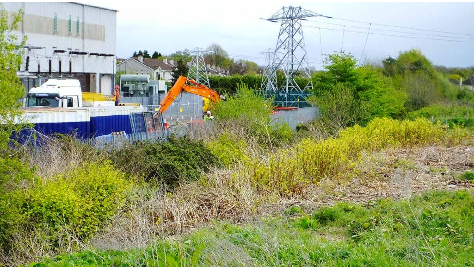
Figure 5.2: Japanese knotweed in close proximity to transmission infrastructure
