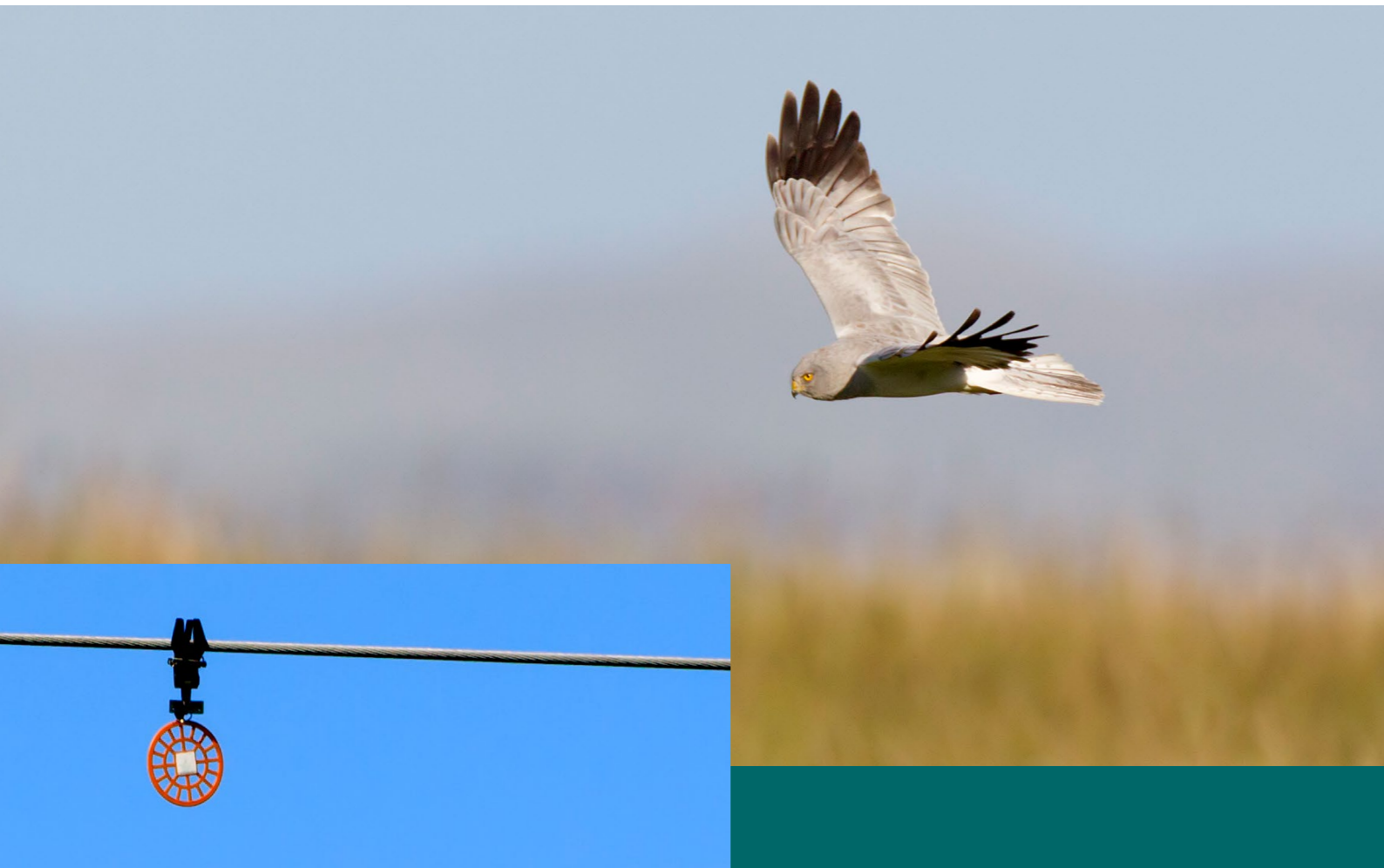
An example of a bird flight diverter installed on an electricity cable.
