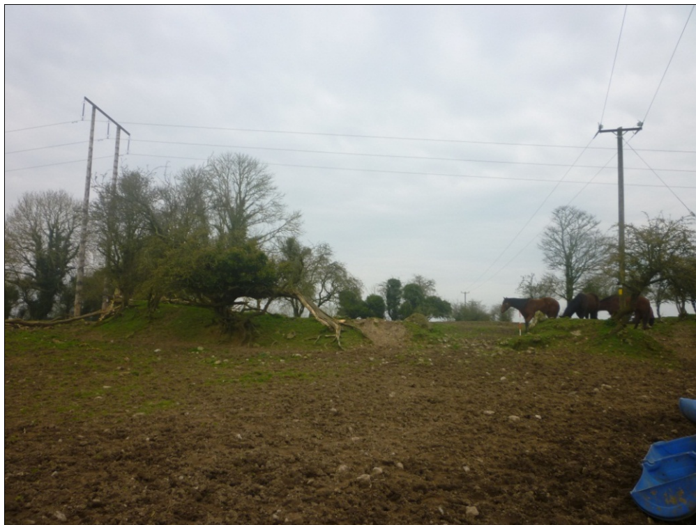
Illus. C 63 Taken from the south, showing 110 kV Lanesboro – Mullingar line and the local connection
