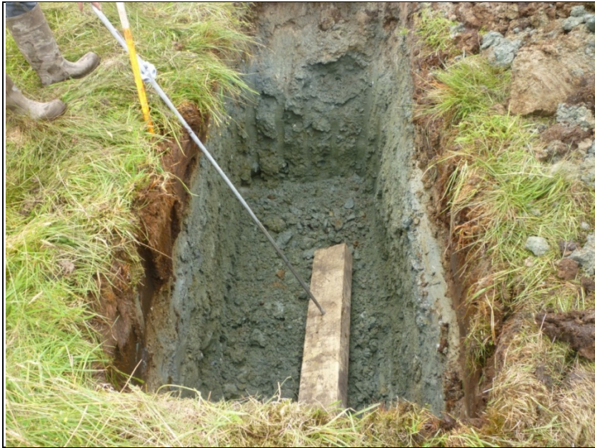
Illus. C 3 Trench required for stay lines, with stay rod in place
