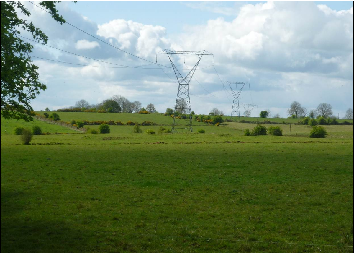
Example of a 220 kV intermediate tower design along the Cashla – Flagford overhead line, Co Roscommon
