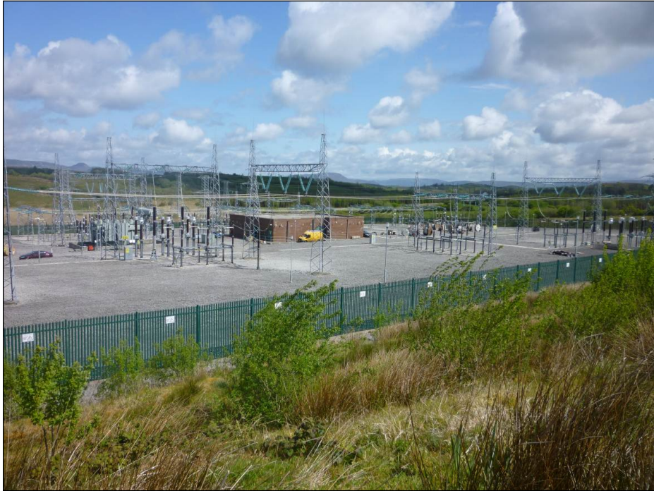
Srananagh 220kV/110kV substation, Co Sligo, example of a typical outdoor AIS substation
