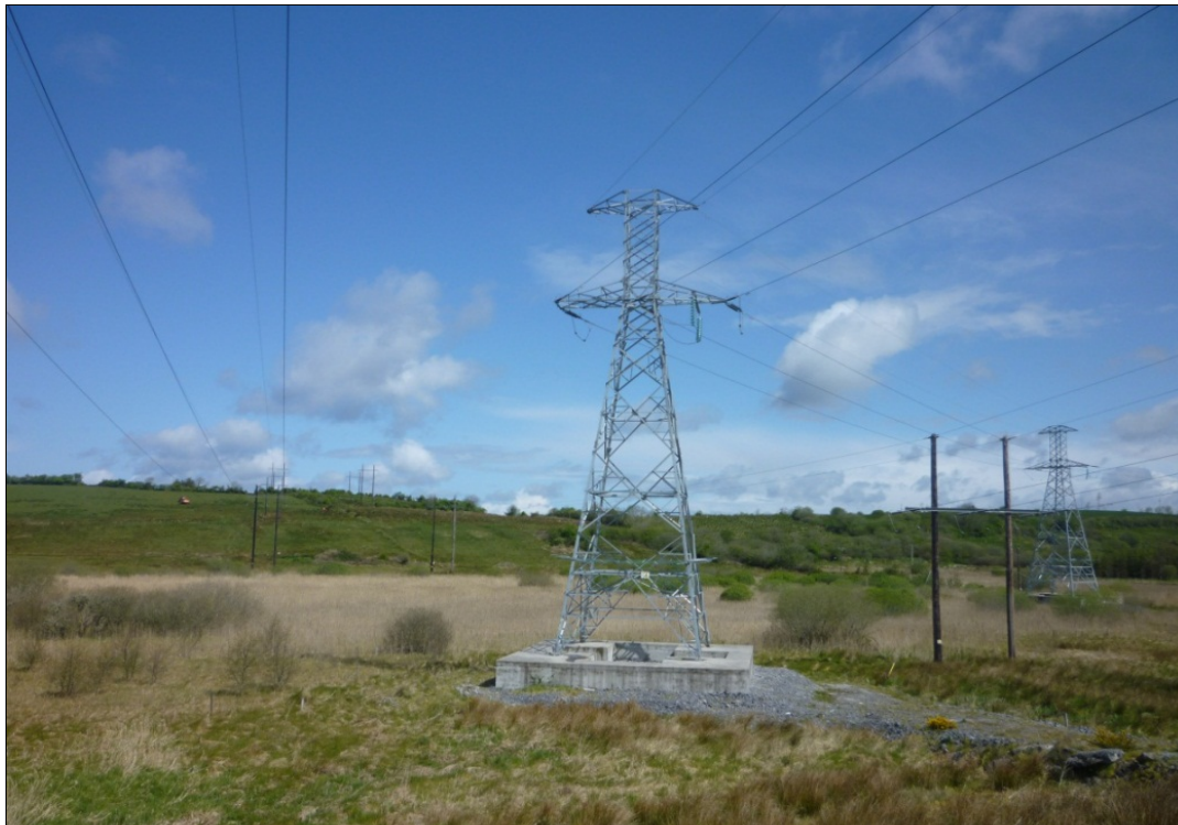
Illus. C 58 North of the substation, steel tower are located in a wetland area (former Castle Lough). The substructure is raised and exposed.
