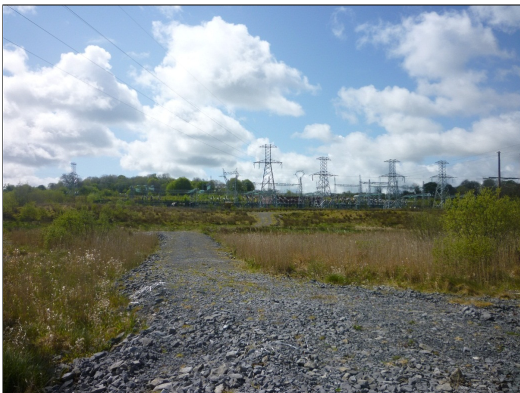
Illus. C 59 Substation taken from the north, woodland (Mullaghbawn Wood) can be viewed in the southeast corner.
