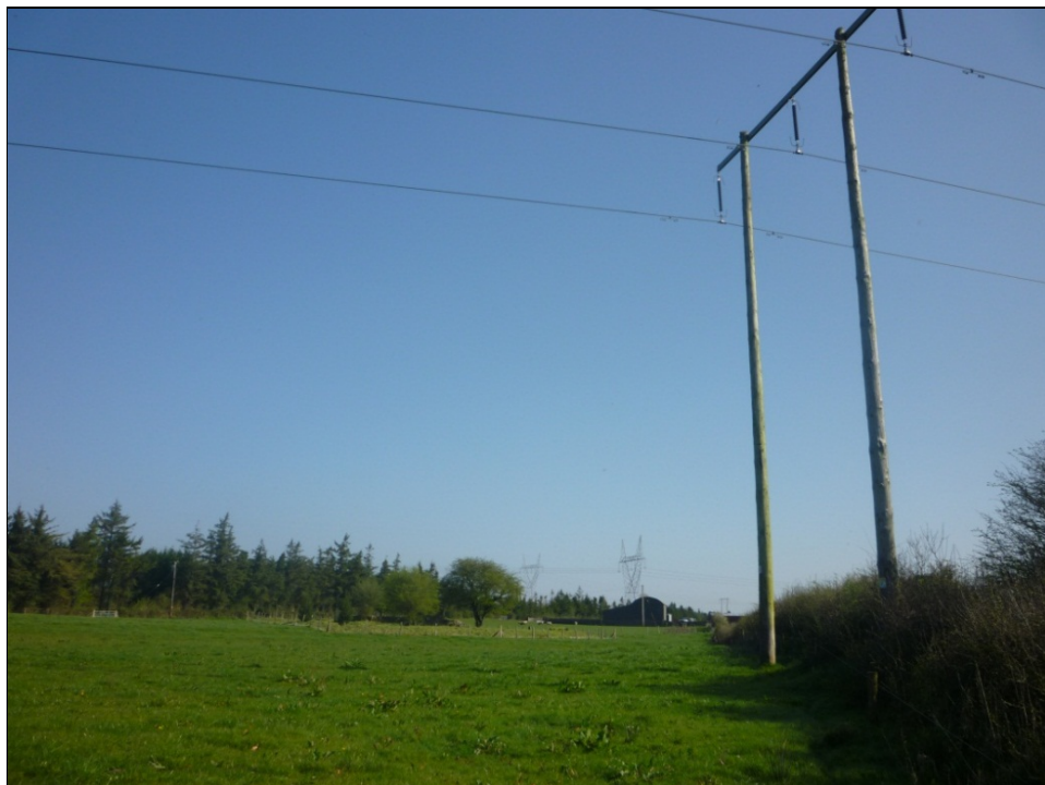
Illus. C 42 Polesets at the field boundary, monument located middle ground and the steel tower in the distance
