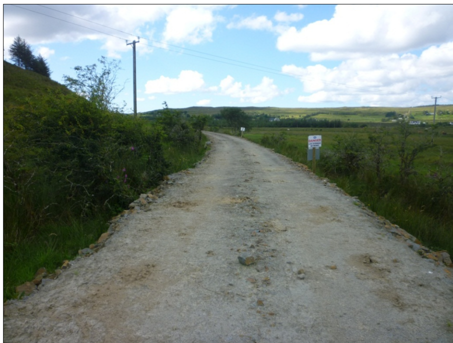
Illus. C 6 New surface of the dismantled railway embankment which acts as an access route
