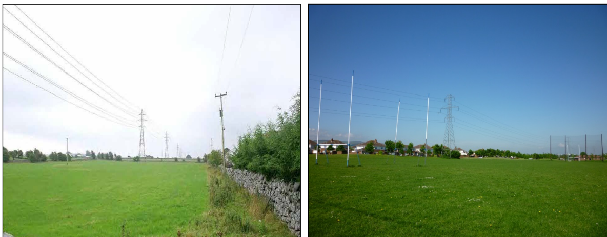
Typical 110 kV double circuit structures
