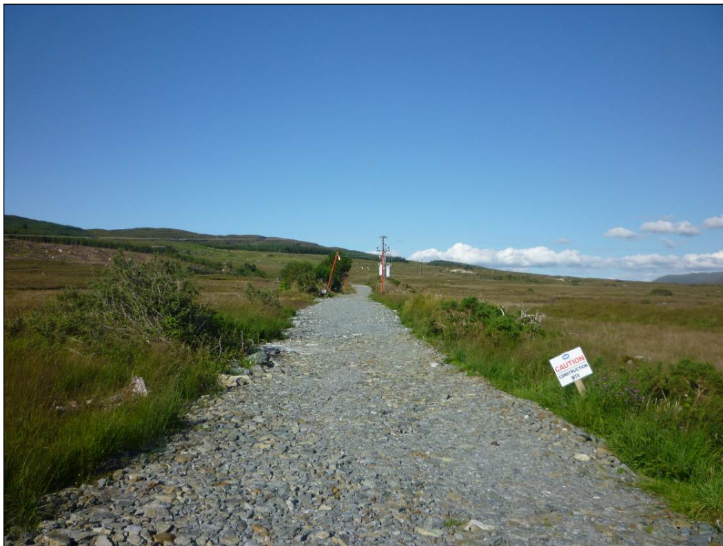
Example of a newly built access route for a transmission project, Co. Donegal
