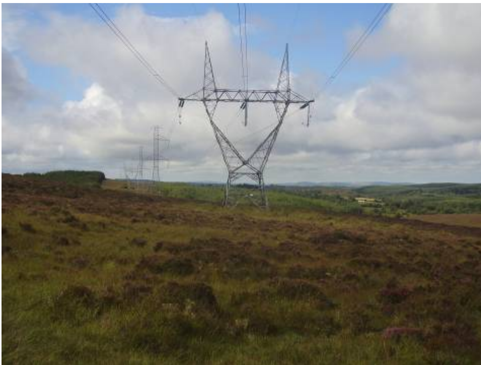
Figure 3.10: Moneypoint to Oldstreet 400kV transmission line showing an example of a 400kV angle tower.
