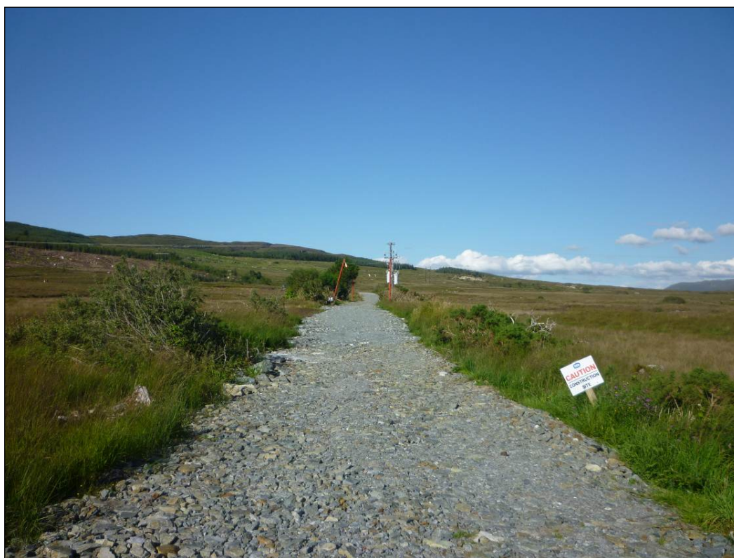
Example of a newly built access route for a transmission project, Co. Donegal
