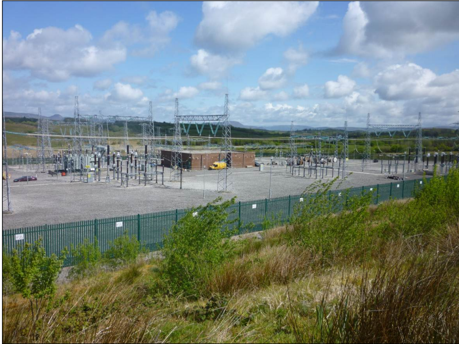
Srananagh 220kV/110kV substation, Co Sligo, example of a typical outdoor AIS substation
