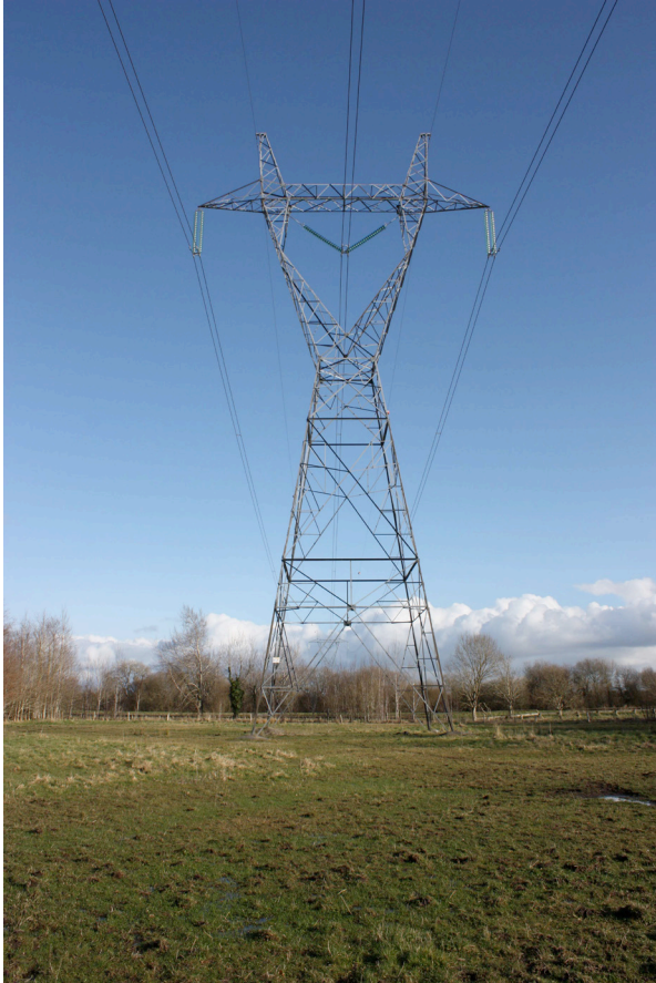
Figure 17b: Study site at Ballymacegan (Oldsteet-Woodland 400kV line)
