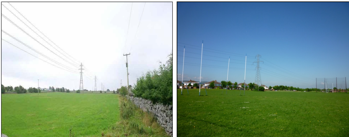
Typical 110 kV double circuit structures
