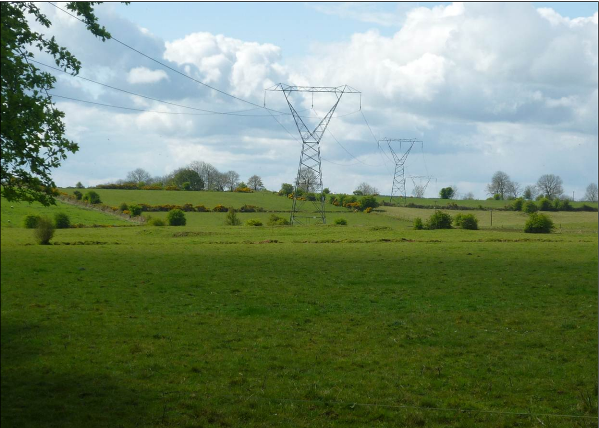
Example of a 220 kV intermediate tower design along the Cashla – Flagford overhead line, Co Roscommon
