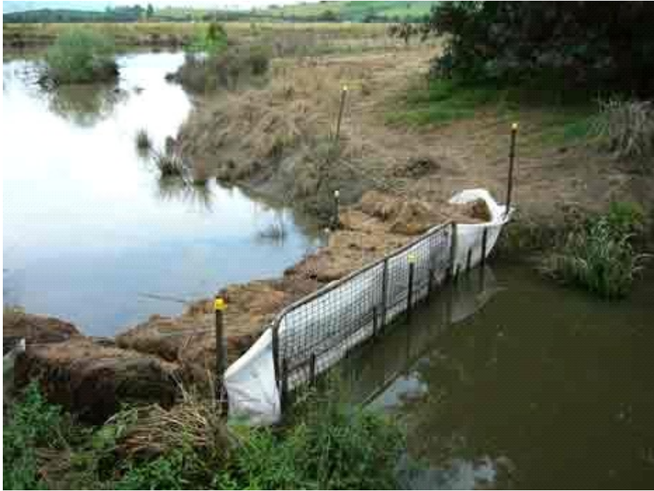
Figure 2.5 Example of straw bales and burlap rolls being used to prevent siltation of river
