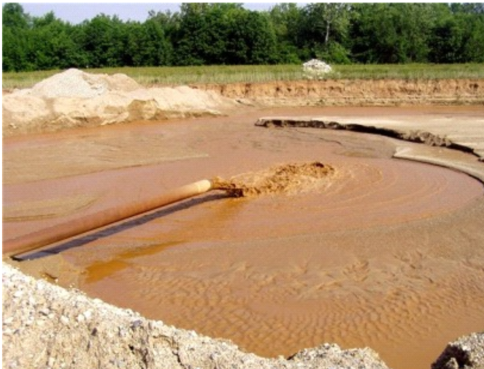
Figure 2.6 Sedimentation pond being used to allow settlement of suspended particles as part of the surface water management of a construction site
