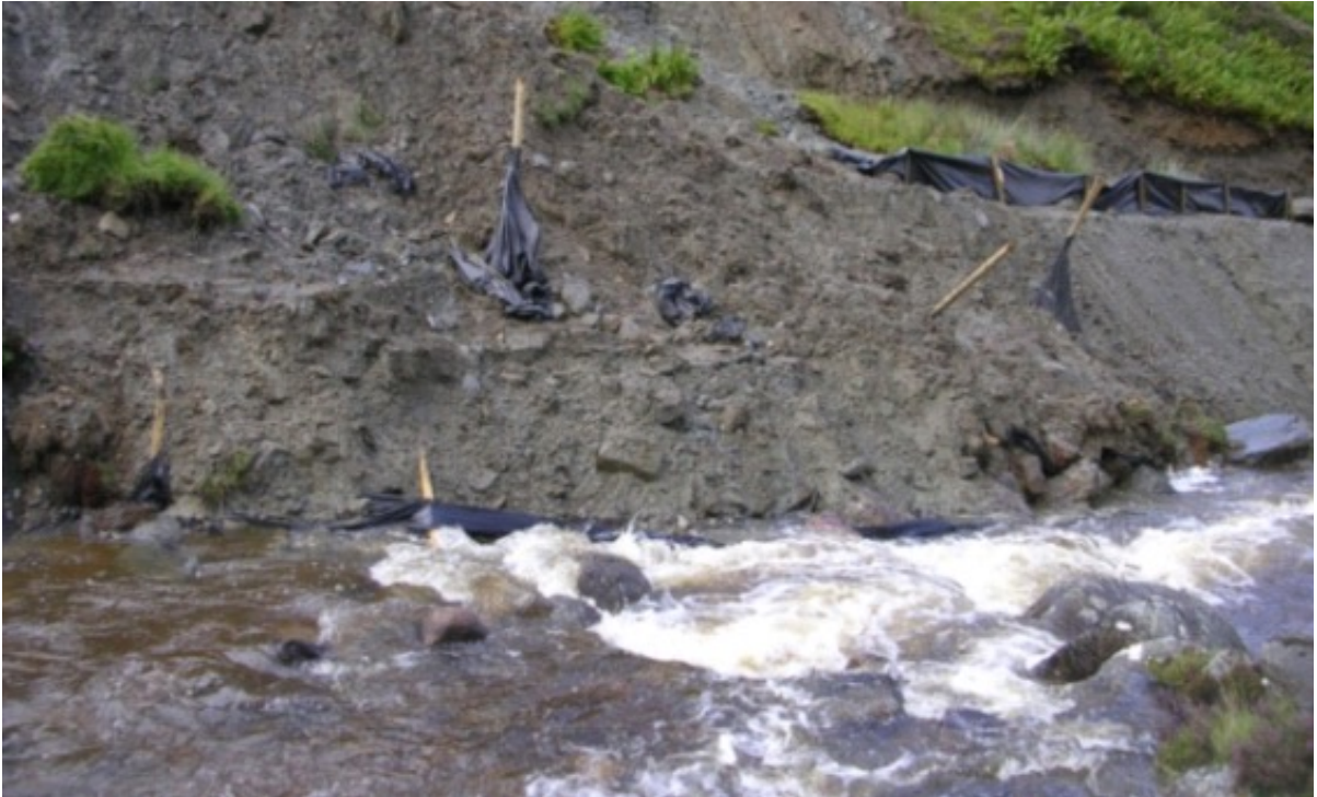
Figure 3.5 Inadequate erosion control measures leading to detrimental damage to adjacent stream
