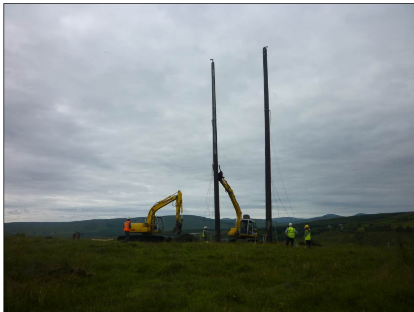
Construction of wooden pole set support structure for Donegal 110 kV Project (Binbane – Letterkenny)
