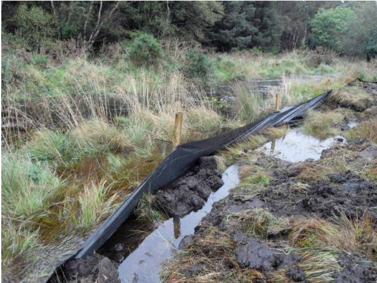
Plate 6.3 Site Clearance works at AM 78 and damage to riparian zone and bank structure
