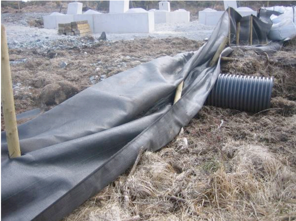
Plate 6.8 Silt fence bypassed by pipe which was a source of peaty silt
