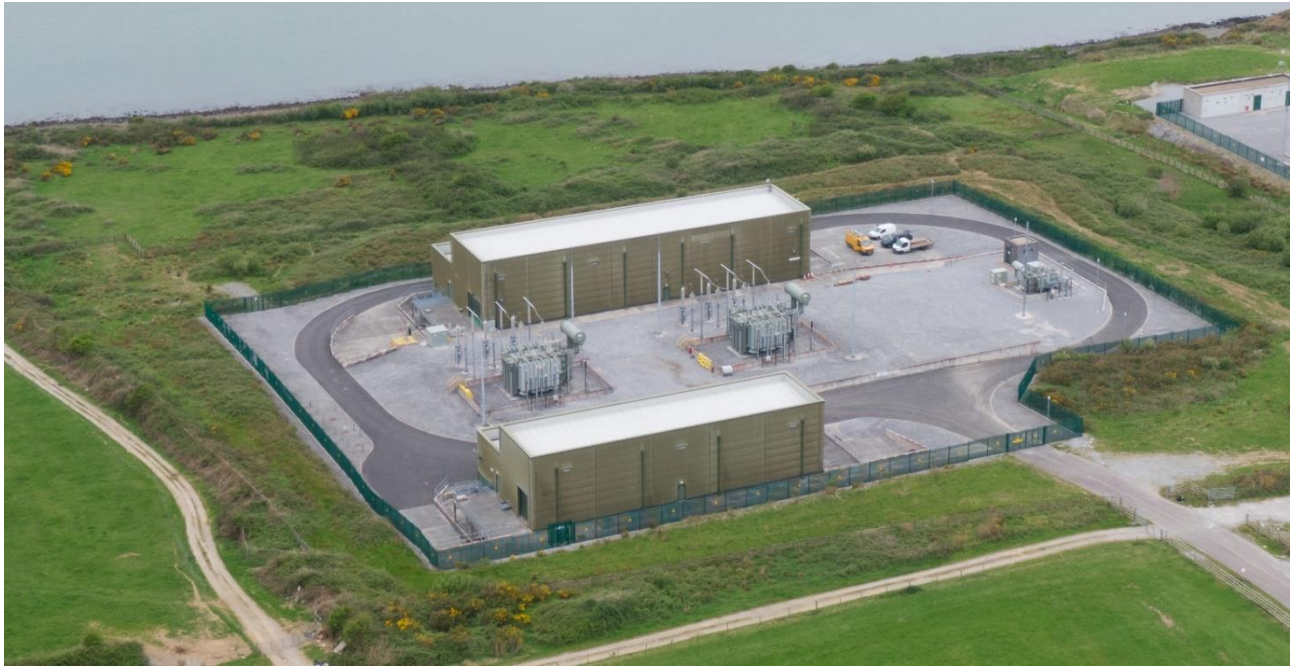
Figure 3-11 - Example of substation with gas insulated switchgear (GIS) – Kilpaddoge 220 kV Substation
