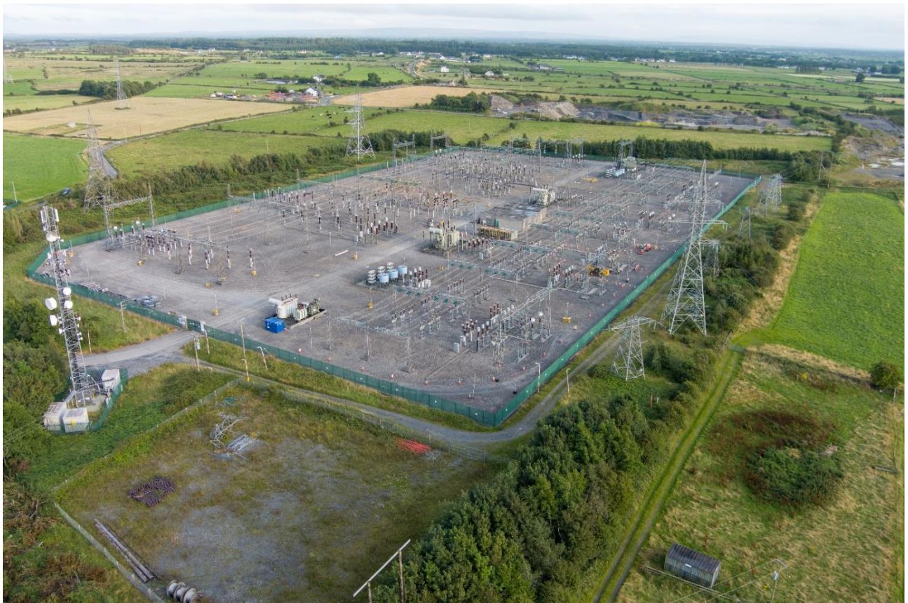
Figure 3-12 - Example of substation with air insulated switchgear (AIS) – Cashla 220 kV Substation
