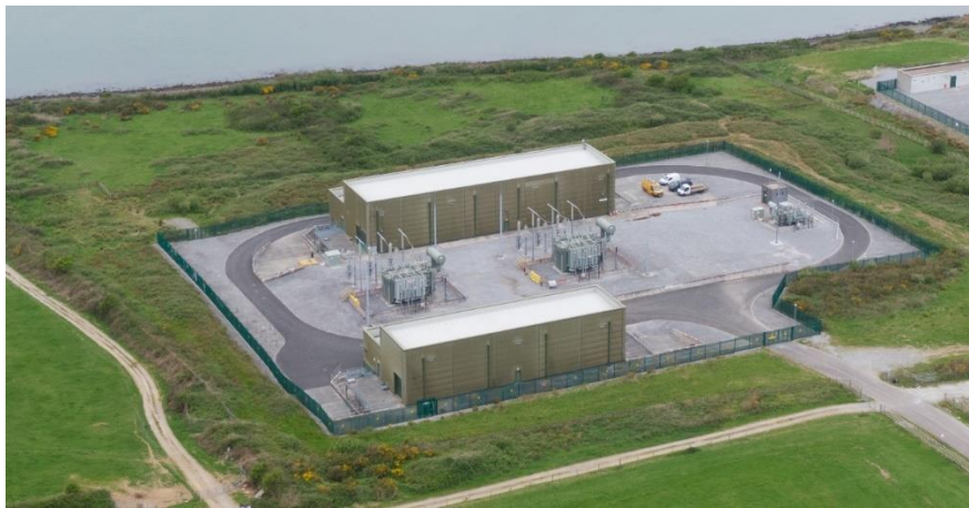
Figure 2. Gas Insulated Switchgear (GIS) Substation
