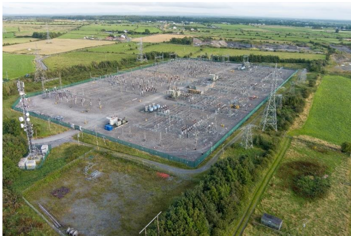
Figure 3: Air Insulated Switchgear (AIS) Substation
