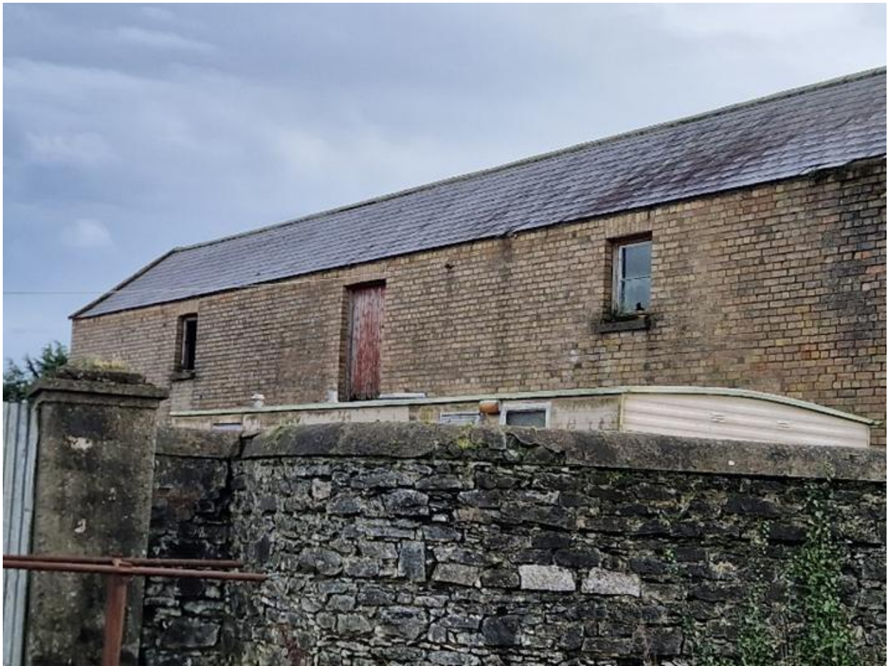
Figure 3-9 - Abandoned building immediately to the east of Site D
