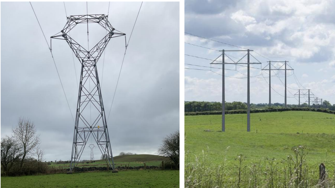
Figure 2.3: Lattice Tower (left) and a Photomontage showing Composite Poles (right)
