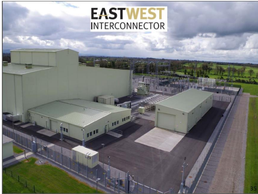
Figure 23 - VSC Converter Station – East West Interconnector [38]
