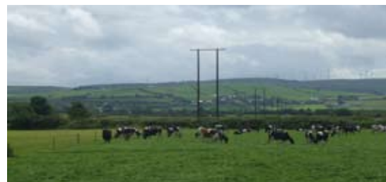
Tarbert - Tralee 2 110kV - Wooden poles
