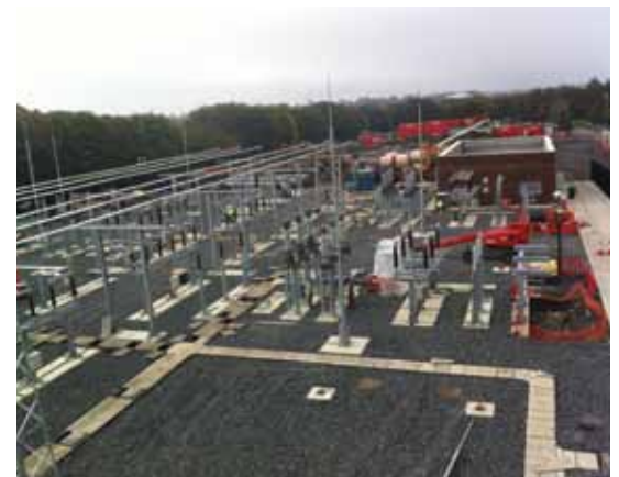
New Cloghran 110kV Station
