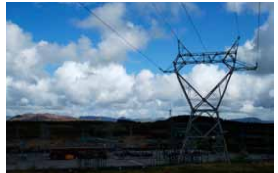
End Mast at Srananagh 220kV Station
