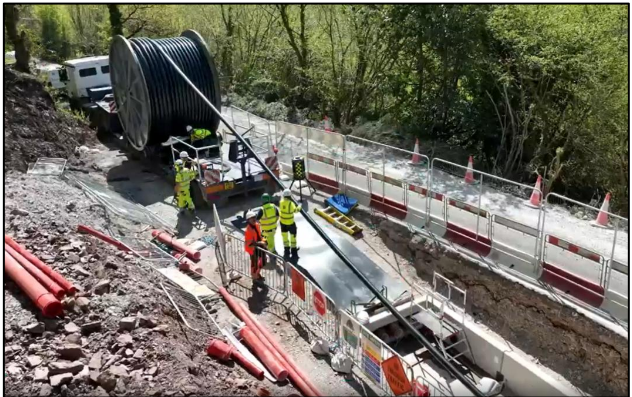
Figure 2-10 - Typical HV UGC laid in ducts / Joint Bay under construction (pre-cast) / Cable pulling (Celtic Interconnector Project)
