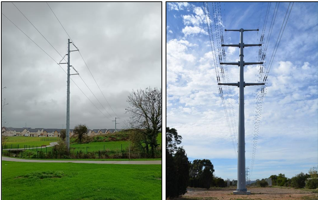
Figure 2-8 - Examples of HV Circuit Steel Monopole Towers (110 kV single circuit and 220 kV double circuit)
