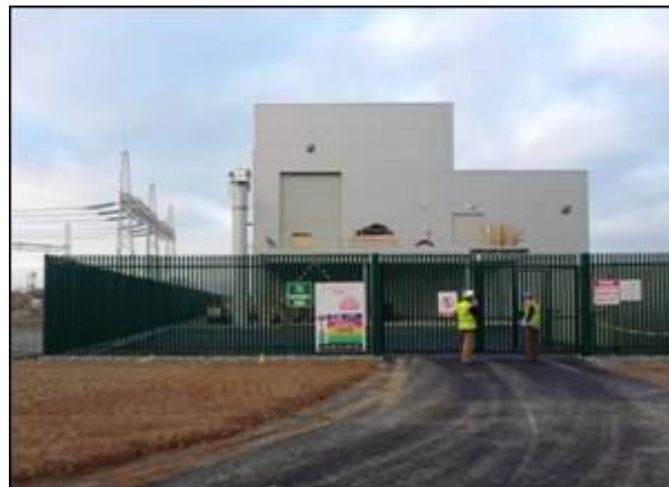
Figure 4-2 Typical GIS Substation
