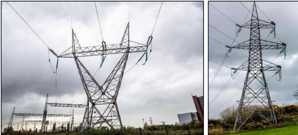
Figure 2-5 - Typical 220 kV OHL Single and Double Circuit Lattice Towers
