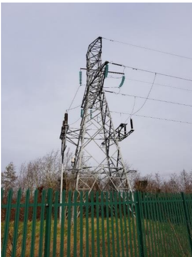
Figure 35: Richmond 2 – Lanesboro Line Cable Interface Mast (LCIM)
