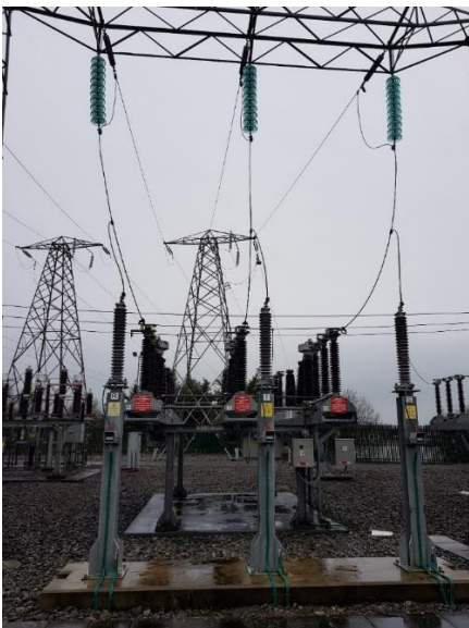
Figure 30: Sliabh Bawn – Lanesboro OHL Termination
