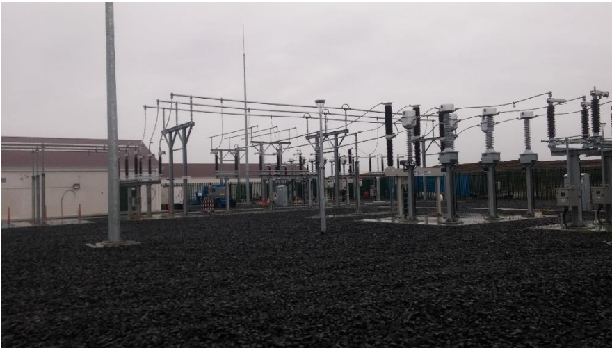
Figure 23: Typical 110 kV AIS Substation
