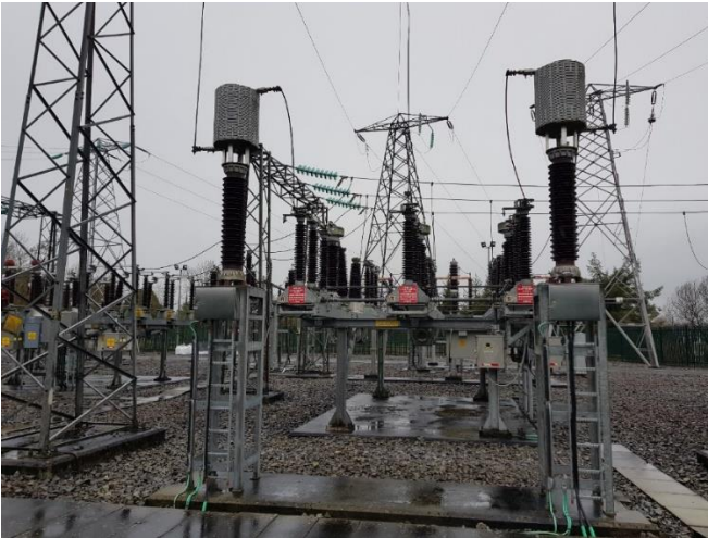
Figure 31: Cloon – Lanesboro OHL Termination
