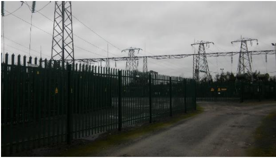
Figure 7: Lanesboro 110 kV Substation
