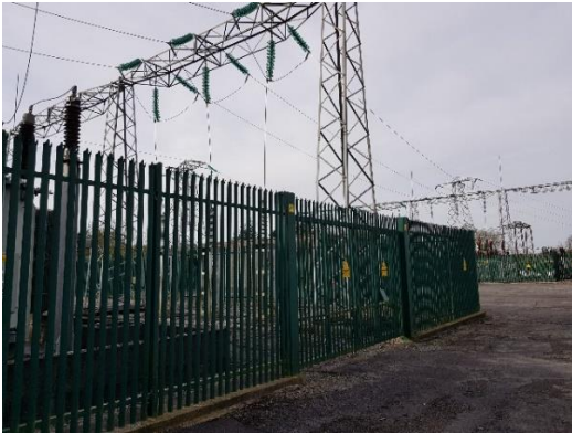
Figure 36: Overhead Line Connection to T141
