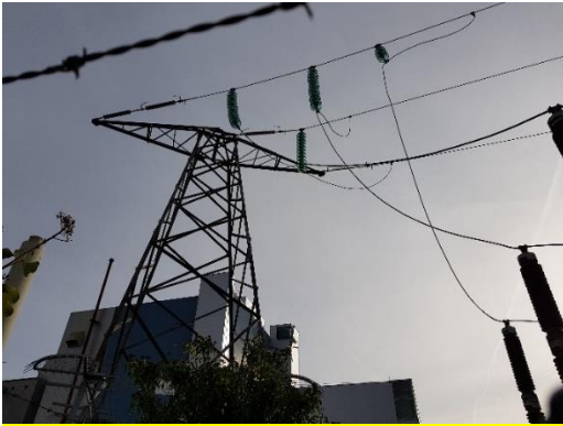
Figure 33: Richmond 1 – Lanesboro Cable Sealing End Compound
