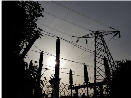
Figure 34: Richmond 1 – Lanesboro Cable Sealing End Compound
