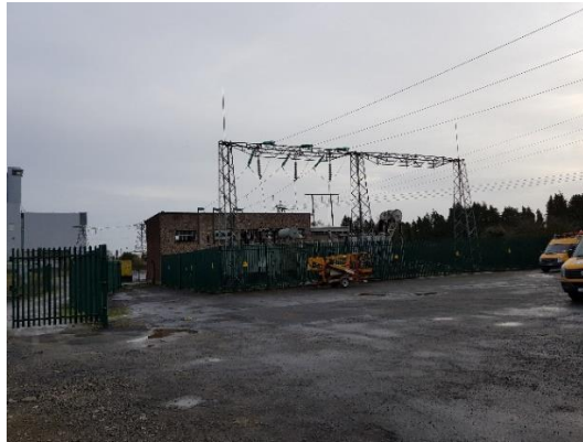
Figure 37: Overhead Line Connection to T141
