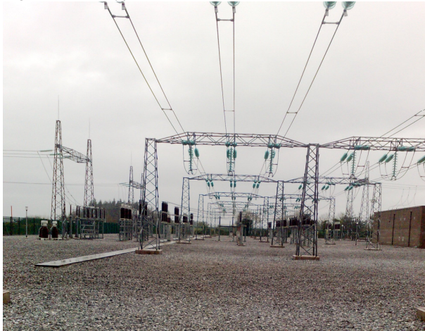
Figure 1.2: Typical AIS Substation
