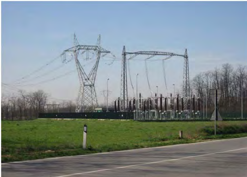
Photo 1: Example of a 400 kV Underground Cable to Overhead Line Transition Station
