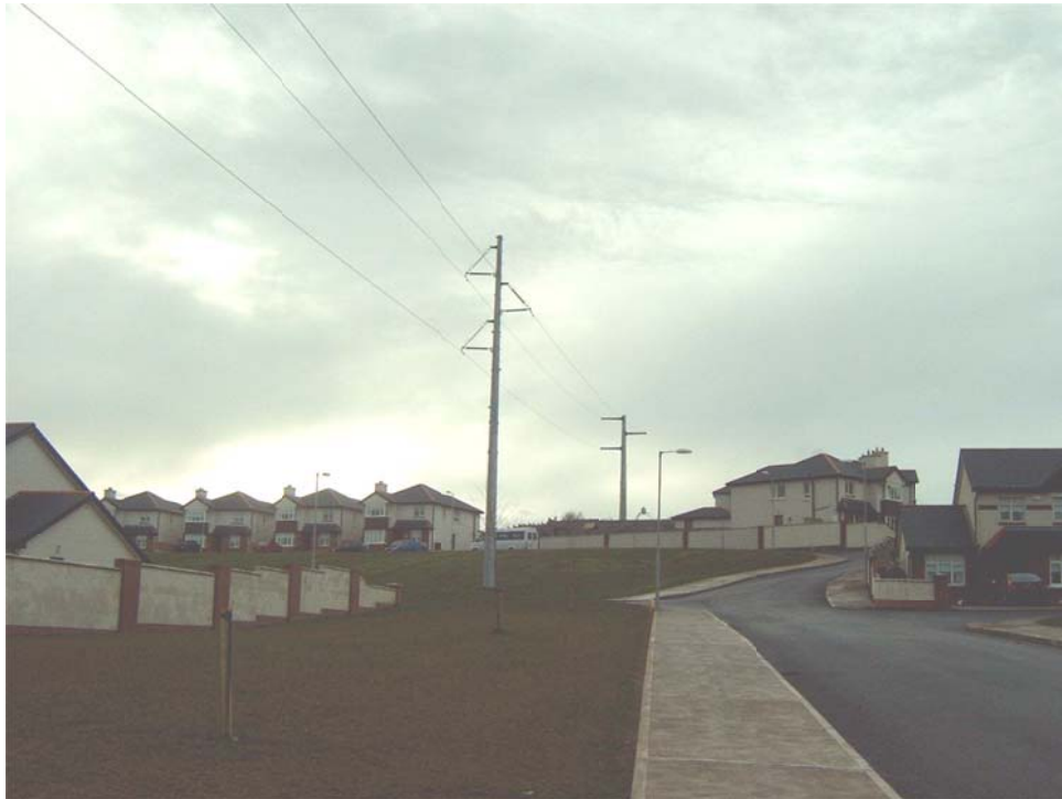
Photo 2: 110 kV Monopole Overhead Line in Cork
