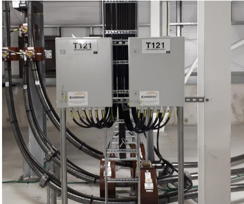
Photo 1 Ring CTs and Metering marshalling kiosk
