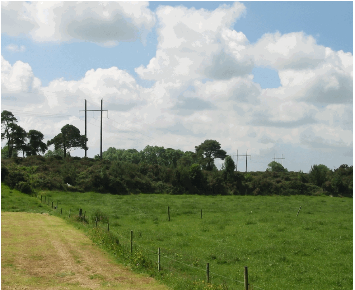
Figure 2: A picture of the earthwire section of the existing Dunmanway-Macroom 110kV Line close to Dunmanway 110kV Station.
