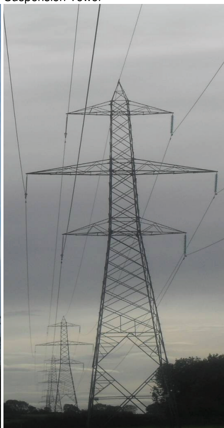
Figure 3.7: Typical 220 kV DC Suspension Tower
