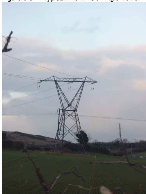
Figure 3.8: Typical 220 kV SC Angle Tower
