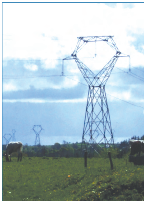
220/110 kV Steel Mast
