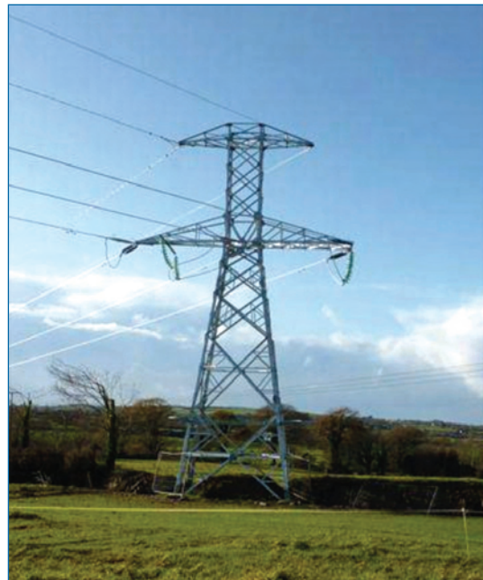
110kV Steel Mast
