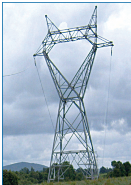
220/110 kV Steel Mast
