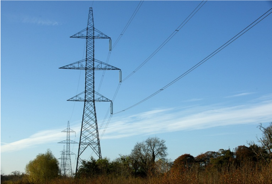
Figure 6.5: Existing 400kV Double Circuit Lattice Steel Tower on the Approach to Dunstown 400kV Substation
