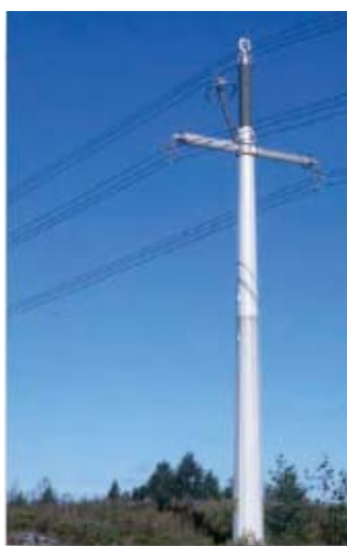
Figure 3: Left 400kV Top Insulated Support Sweden (in service)
