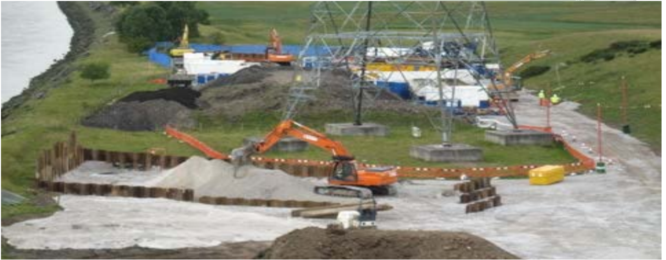
Figure 3.10 – Example of compound size and working area required for Horizontal Directional Drilling (HDD)
