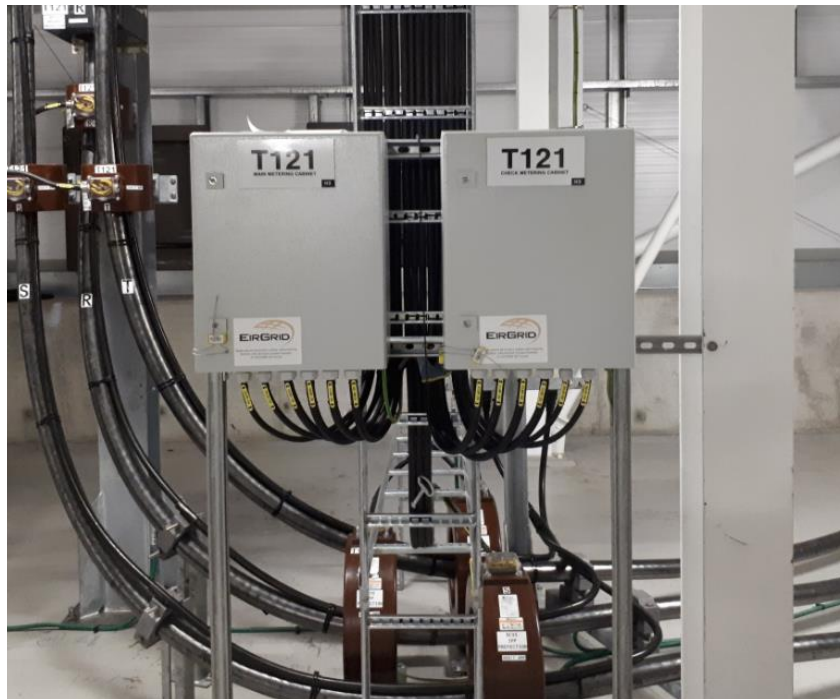
Photo 1 Ring CTs and Metering marshalling Boxes
